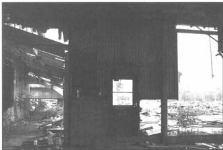
Some abandoned buildings are more hole than wall.
