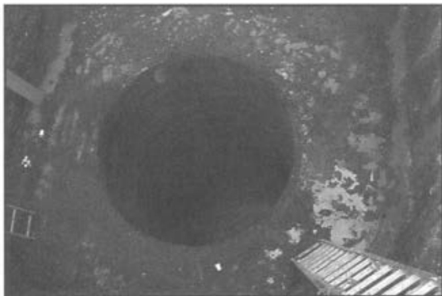
There are no guardrails at most construction sites, so watch out for deep pits.
