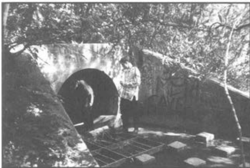
In some cases, grates to drain outfalls have been completely removed.
