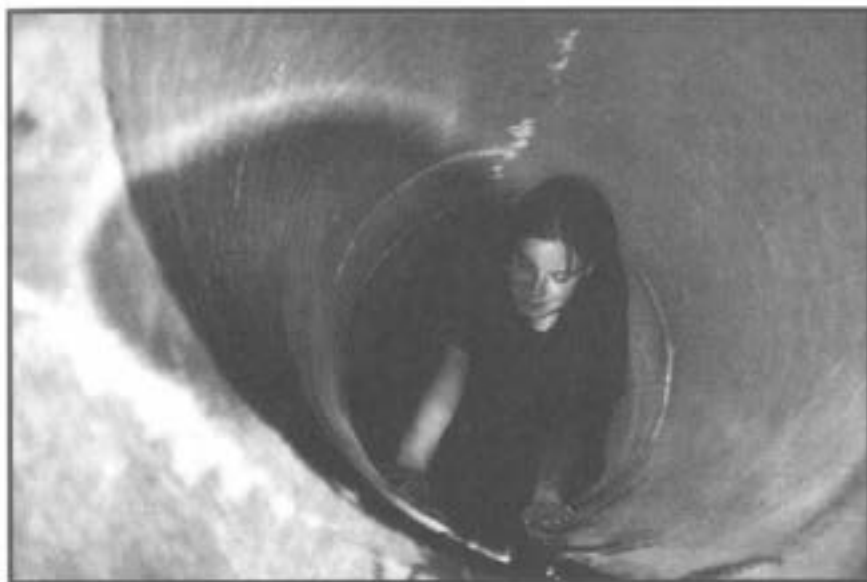
Small sidepipes in drains are often humanly accessible but not comfortable.
