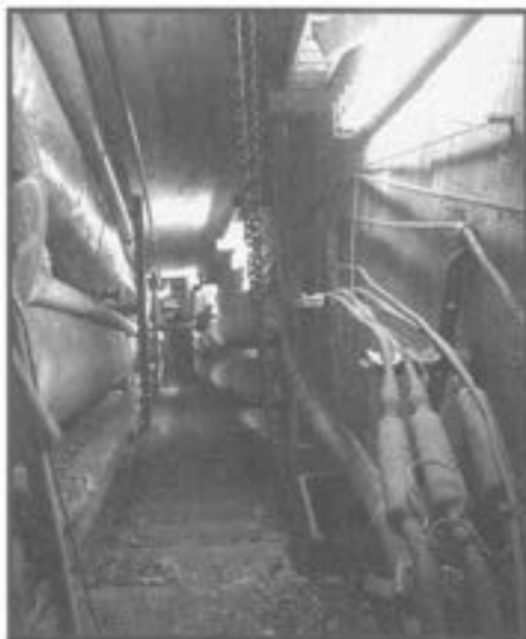
Sometimes utility tunnels change elevation drastically or even span over multiple levels.
