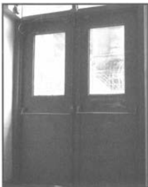
These supposedly alarmed doors are sitting slightly ajar, indicating that the alarm isn't doing much.
