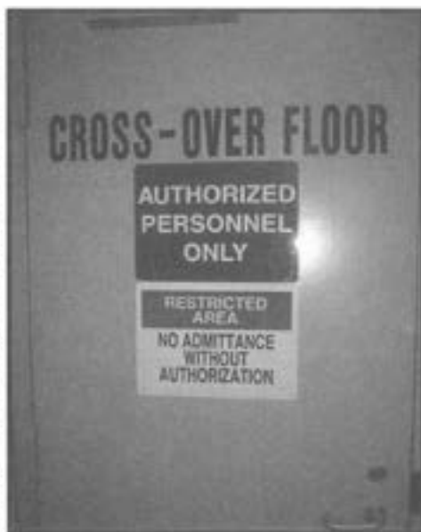
Crossover floors, whatever their signs may warn, should be unlocked in compliance with fire codes. They're good routes out of stairwells.
