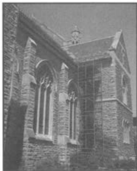
Scaffolding can provide a handy route up or down at renovation sites.
