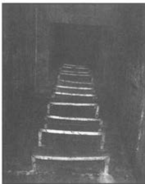
Stepirons set into the concrete at the side of the drain are often used in place of ladders.
